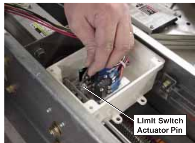
Photo 5 - Center limit switch actuator pin between limit switch arms.
